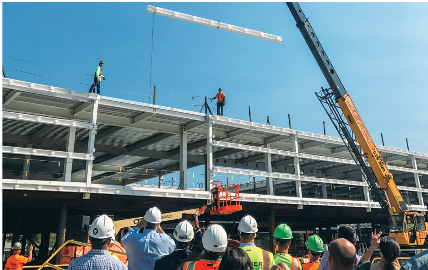
A crowd watched as the final steel beam was put into place for the Ed Kaplan Family Institute for Innovation and Tech Entrepreneurship. Illinois Institute of Technology donors, faculty, staff, students, and alumni were joined at the September 15 event by key local officials including Mayor Rahm Emanuel. Watch a livestream of the construction site at http://bit.ly/2vtbVyQ . Photo: Denise Moriarty
