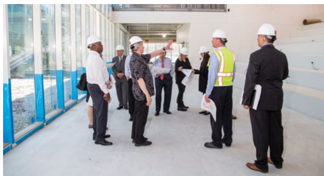
Howard Tullman, executive director of the Ed Kaplan Family Institute for Innovation and Tech Entrepreneurship [center], led a tour of the construction site for members of Illinois Tech's Board of Trustees in May. Photo: Michael Goss
