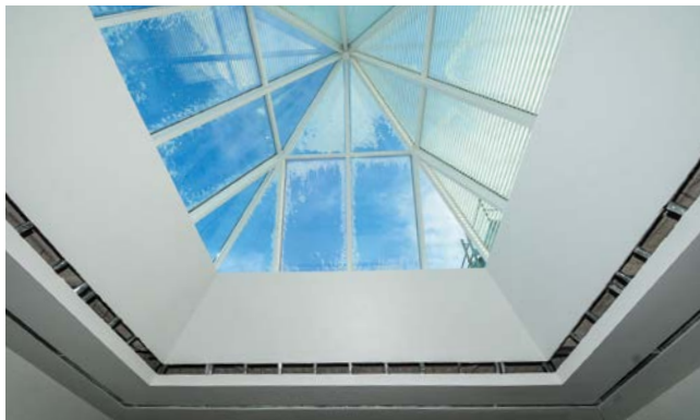
One of three brand-new skylights toward the north end of E1, which will fill the atrium space below with light
