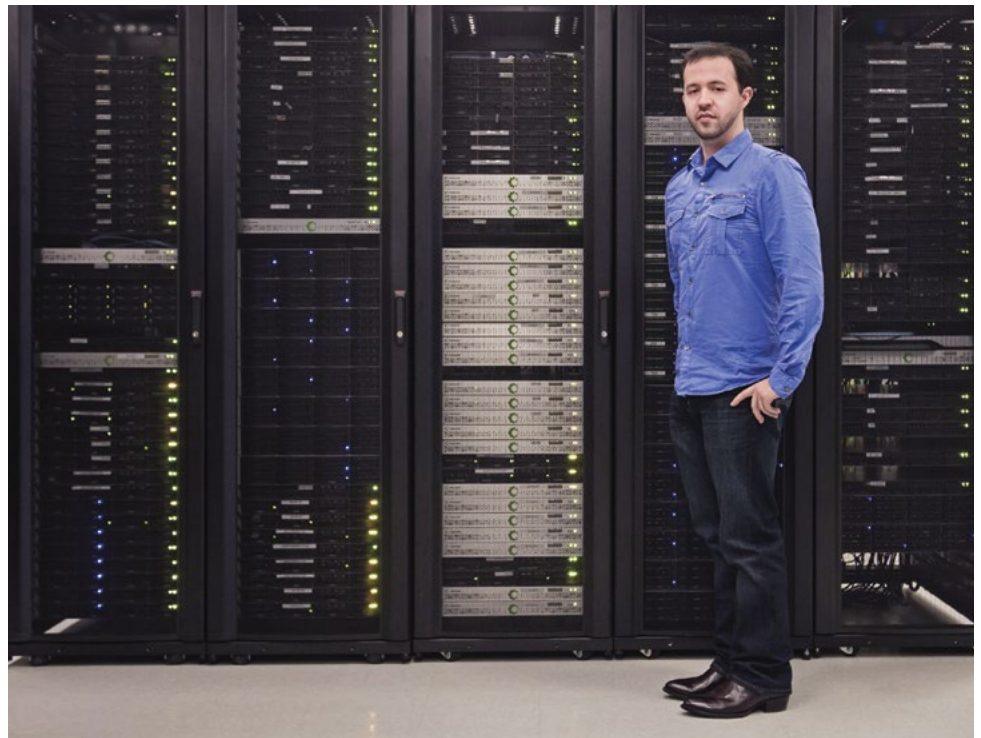
IIT alumnus Jason Resch stands by a Cleversafe data center in the Chicago office. The center contains rows of server racks, each of which contains up to 40 separate computers, and is used for internal testing, development, and research purposes.
